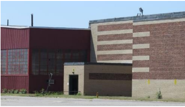
Fig. 4. East side of the Simonds Saw factory and a corrugated metal-enclosed shed (left).
