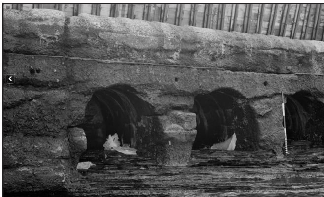
Figure 6. Southwest facing view of the Romanesque Arches. (Historic American Engineering Record, 1968, Library of Congress.)
