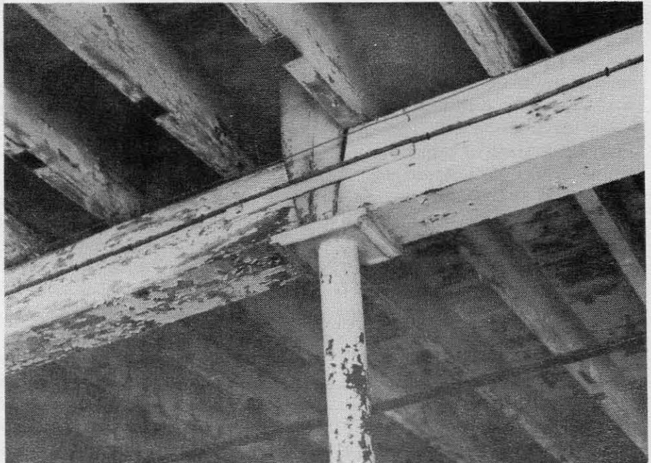
Detail of floor supports of the Somersworth Building Co. shoe factory. Probably for reasons of economy, the builders did not employ "slow-burn" construction. Photo taken in addition (structurally similar to original part).
